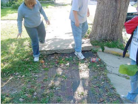
Uneven and missing sidewalk sections interfere with mobility
