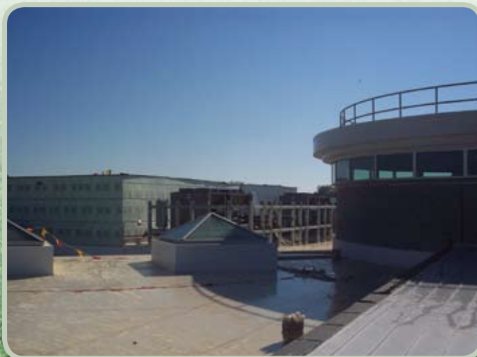
▲ Early construction of the facility rotunda, which is the central point of the Secondary Center.
