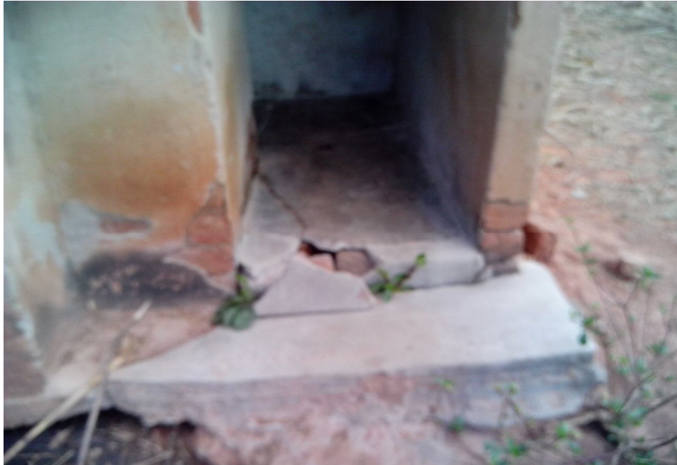
Figure 1. School Blair toilet with narrow entry.
