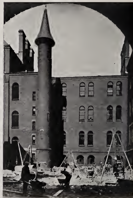
The Boston English High School—oldest in America—built in 1821, is being reconstructed and provided with an addition by a Public Works Administration grant. Largest of Boston's secondary schools with 3,700 pupils, it was originally known as the English and Latin School.
