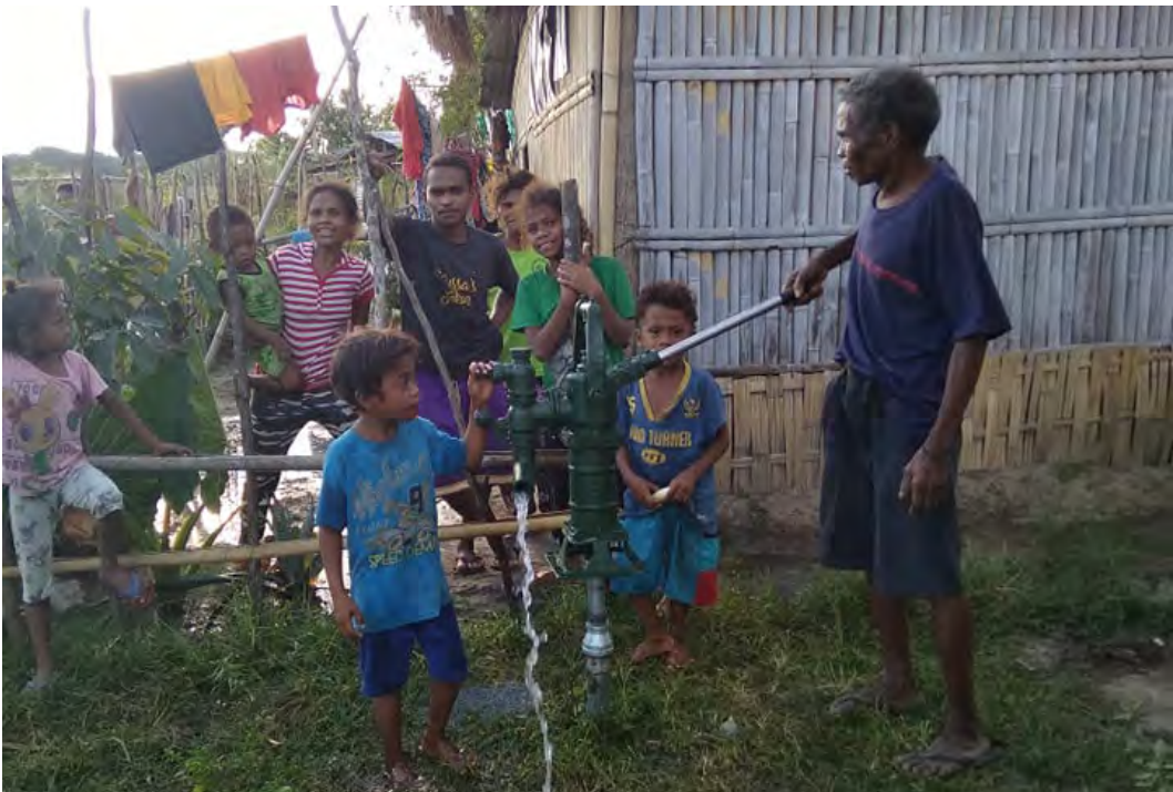
Figure 3. Jetmatic Water Hand Pump Installed for Use by Aeta Families
