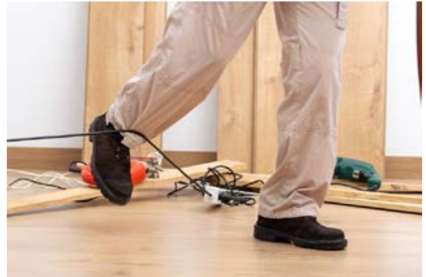
Extension cords create common trip/fall hazards.
